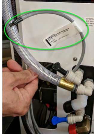
5 Conductor wire: Tank Full Switch, Green + Orange
